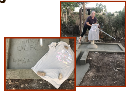
An Example of a Newly Installed FFL Public Clean Water Well in Fort Liberté, Haiti with Business Sponsorship Recognition (November 2018)
